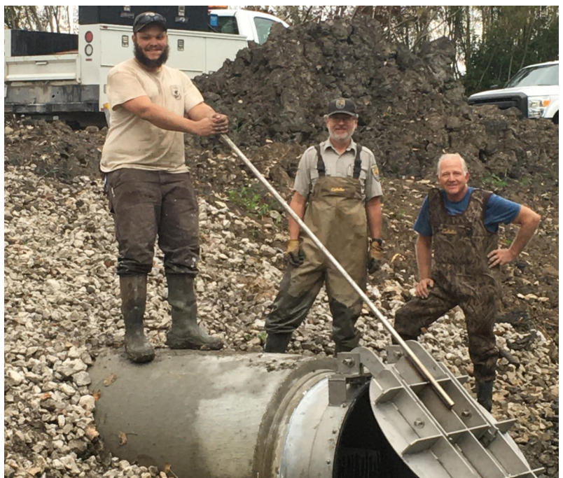
Maintenance Worker Ramsay Houze, Refuge Biologist Ron Huffman, and FWS volunteer Mike Bohling work together to replace water control structures at the Darby Unit near Port Clinton, Ohio.
